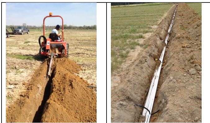
Figure 4. (a) Digging a trench with a trencher, and (b) water supply lines inside one of the trenches.
