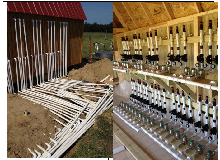
Figure 5. (a) Water supply lines connected to SDI control center, and (b) control manifolds for each plot.
