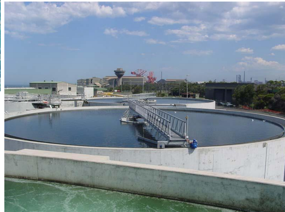
Clarifier in Water/Wastewater Treatment Plants
