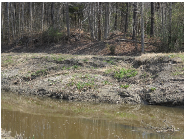
Figure 2. Bank failure is a symptom of stress.
