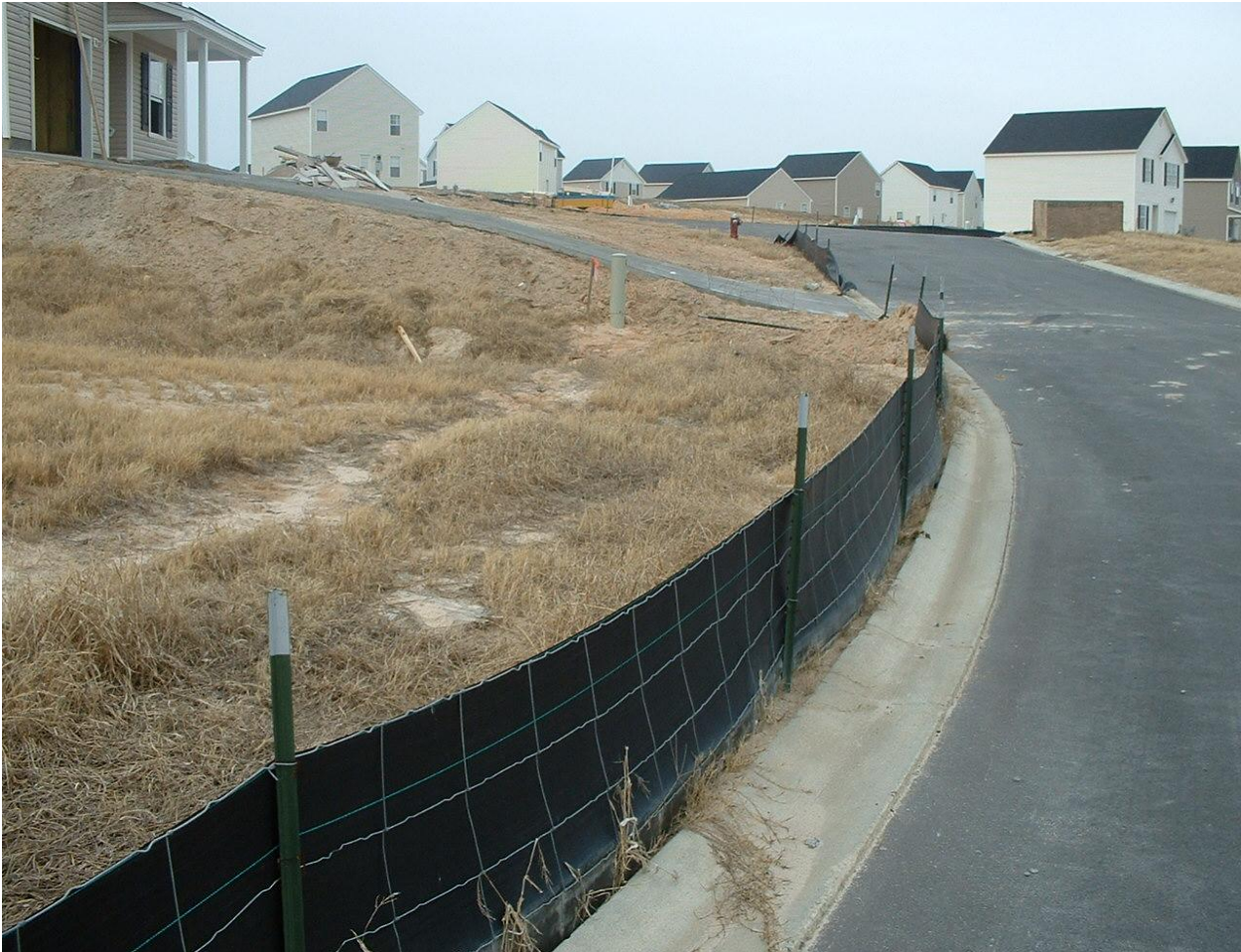
Figure 1: Use of silt fence on a residential lot under construction in study area
