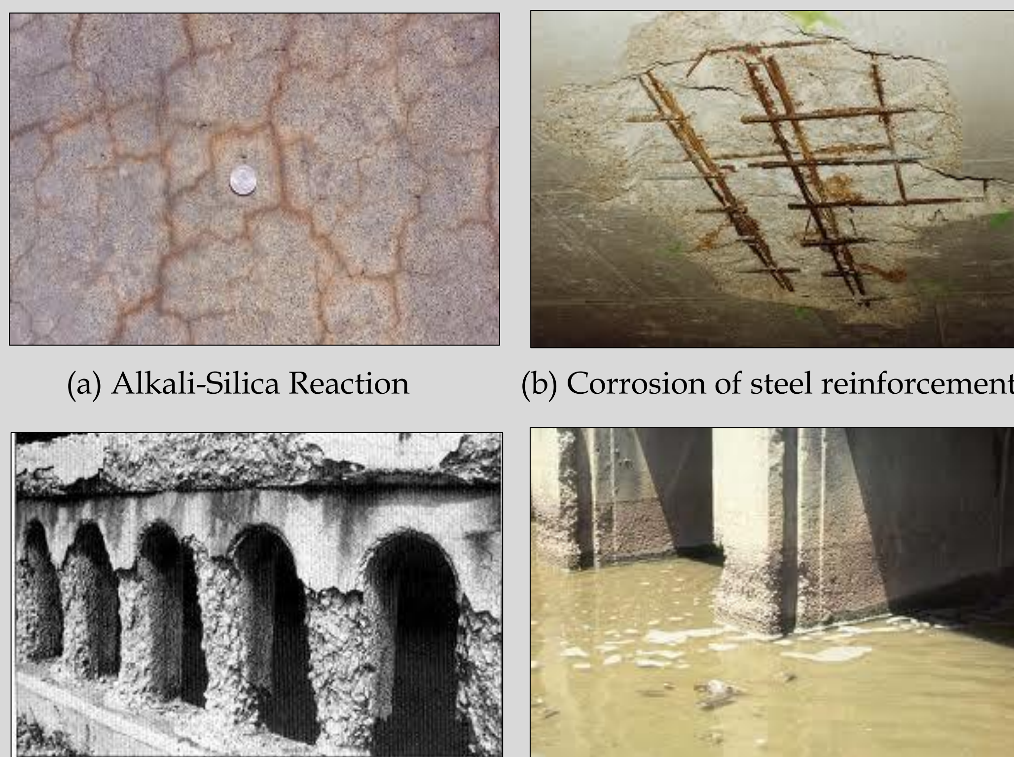
Figure 1: Major durability problems in concrete structures
