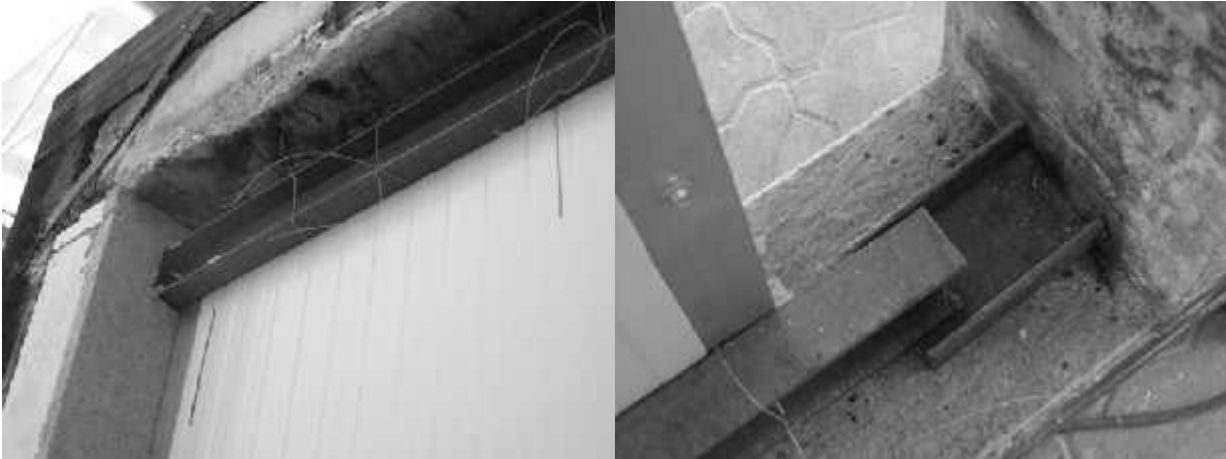
Fig. 3 The load-bearing steel structure was allowed to expand during the fire resistance test (simulation of a situation that the wall installed in practice will be wider than the 3m tested width)
