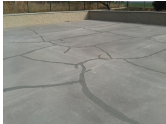
FIGURE 1. The example of cracks propagation due to shrinkage.
