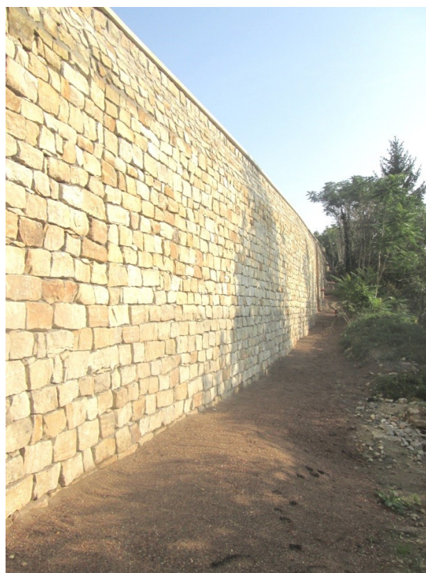
FIGURE 3. Structural condition comparison: the old (top) and the new wall (bottom).
