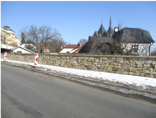
FIGURE 2. View of the original (top) and new wall (bottom) near St. Barbara's dome.
