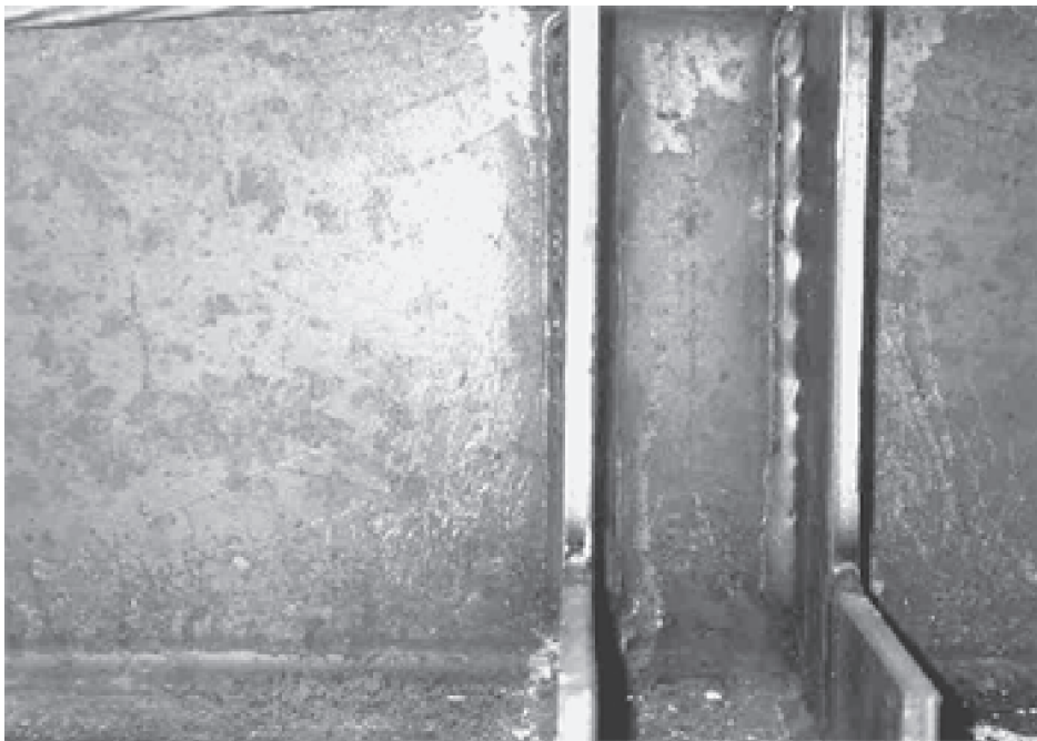
Fig. 7: Diagonal flaking of mill scale indicating the yield development about the inner support section
