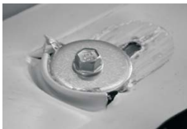
Fig. 6: The collapse mode of the connection from set B, temperature 200 °C
