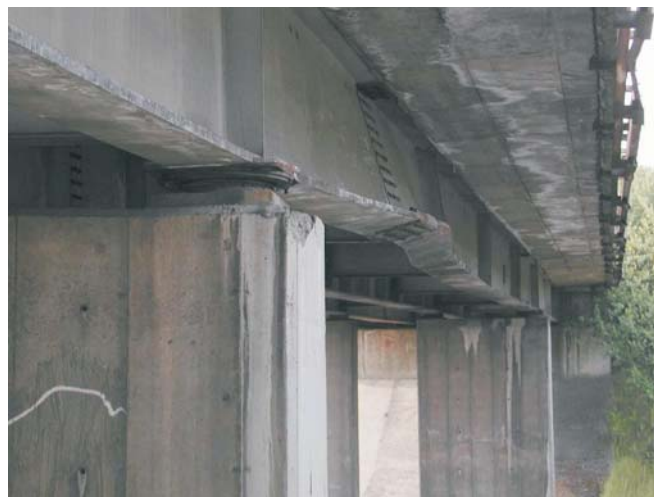
Fig. 6: View of the damaged main girder of the bridge
