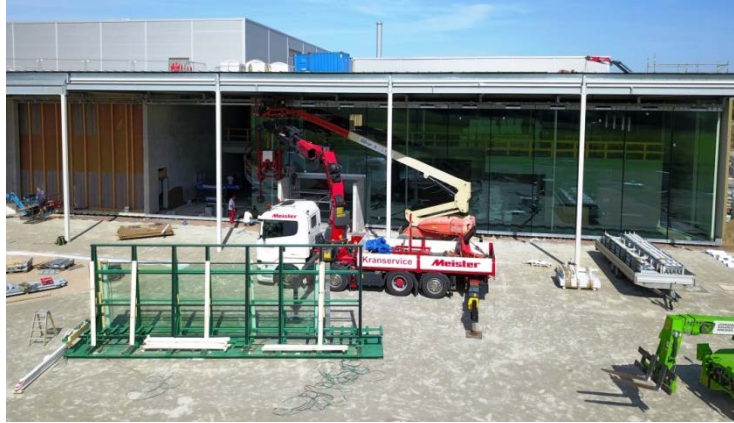
Fig. 6 View of the construction site of the filter factory Wilsdruff during the glazing process.
