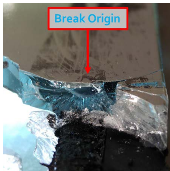
Figure 2. Ceramic enamel frit opacifier on spandrel glass with the thermal stress fracture located where frit material interfaces with glass.
