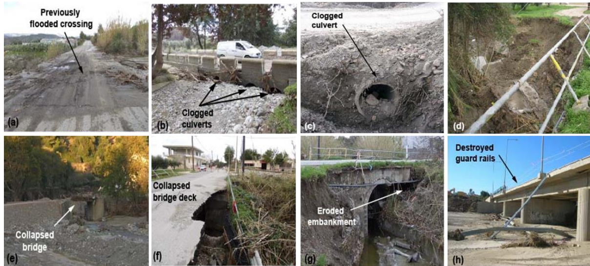
Figure 6. Types of damages on river crossing infrastructure, ranging from inundation only (a), clogging of waterways (b, c), damages on parts of a bridge (d, f, h) and complete collapse of the infrastructure (e, g)
