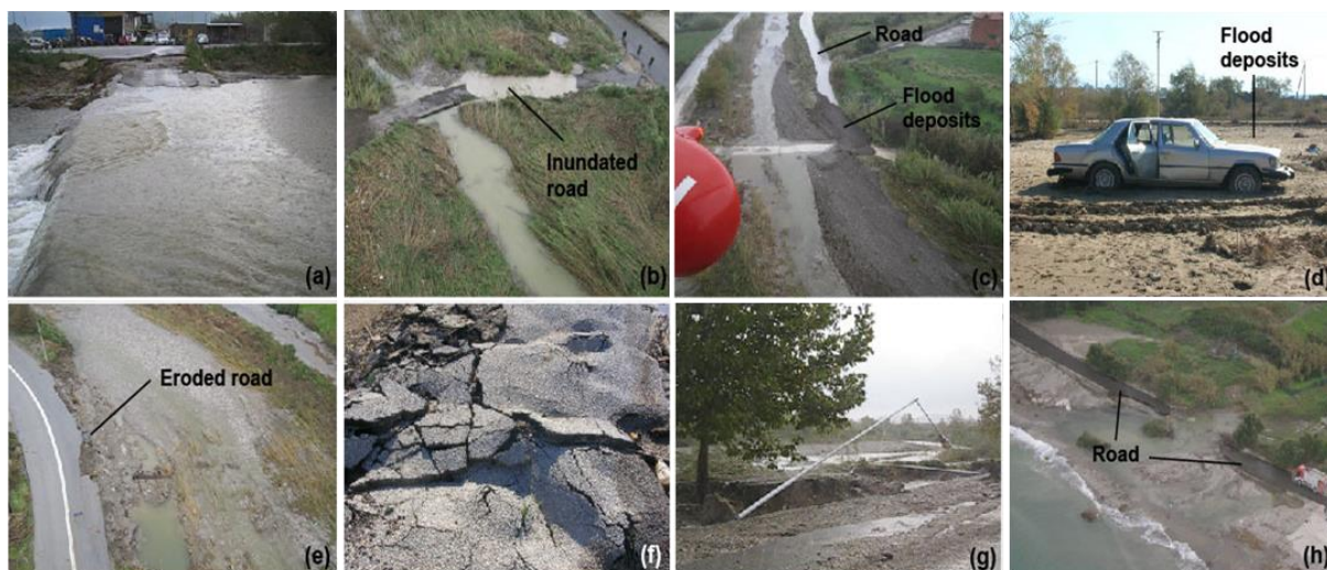
Figure 4. Effects of flash flooding caused by extreme precipitation events on the road network including: inundated parts (a, b), deposits of debris (c, d), eroded road fill and scoured roads (e), asphalt scouring (f), damages on road equipment (e.g. lighting installations) and (g) complete erosion and road collapse (h)
