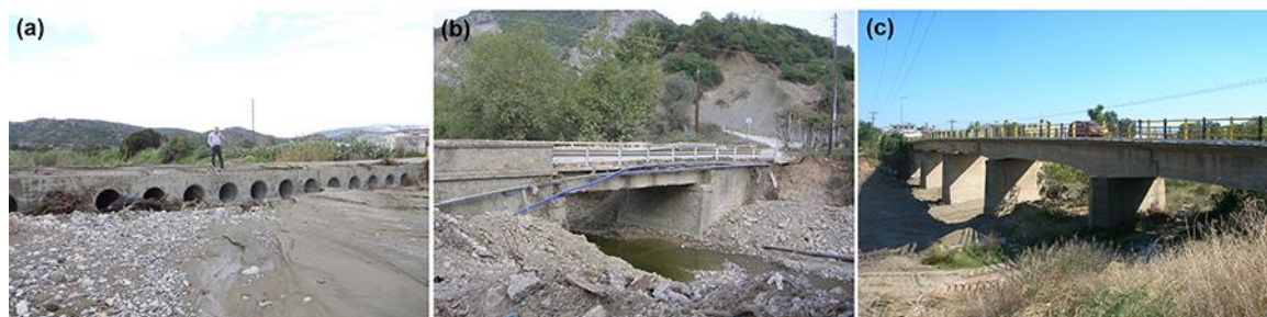
Figure 2. Types of river crossings: (a) low water crossings, (b) single-span bridges and (c) multi-span bridges
