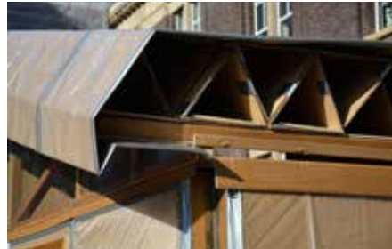
FIGURE 7.43 Inlets of the tropical roof
