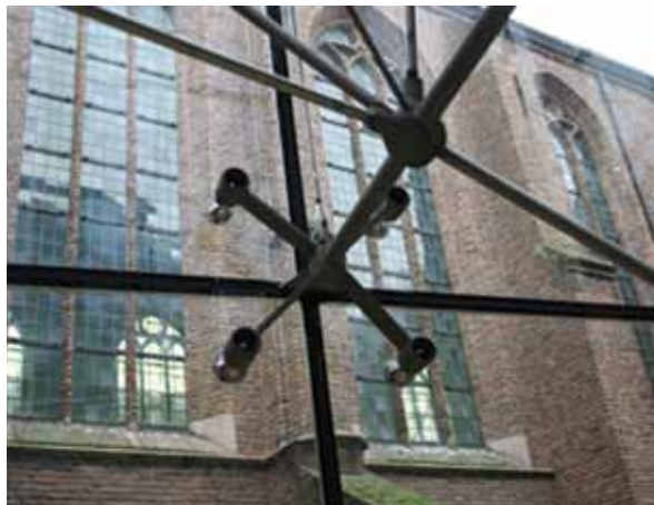
Figure 74 Frameless facade system. The Glass panes are held by a steel 'spider' (Prinsenhof, Delft, Octatube).
