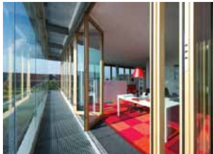
Figure 146 The picture shows the façade cavity with the inner insulated leaf opened.
