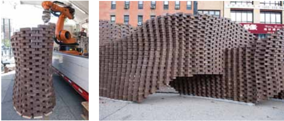
Figure 140 Onsite fabrication of the Pike Loop Installation. It is a self supporting double curved installation in New York.
