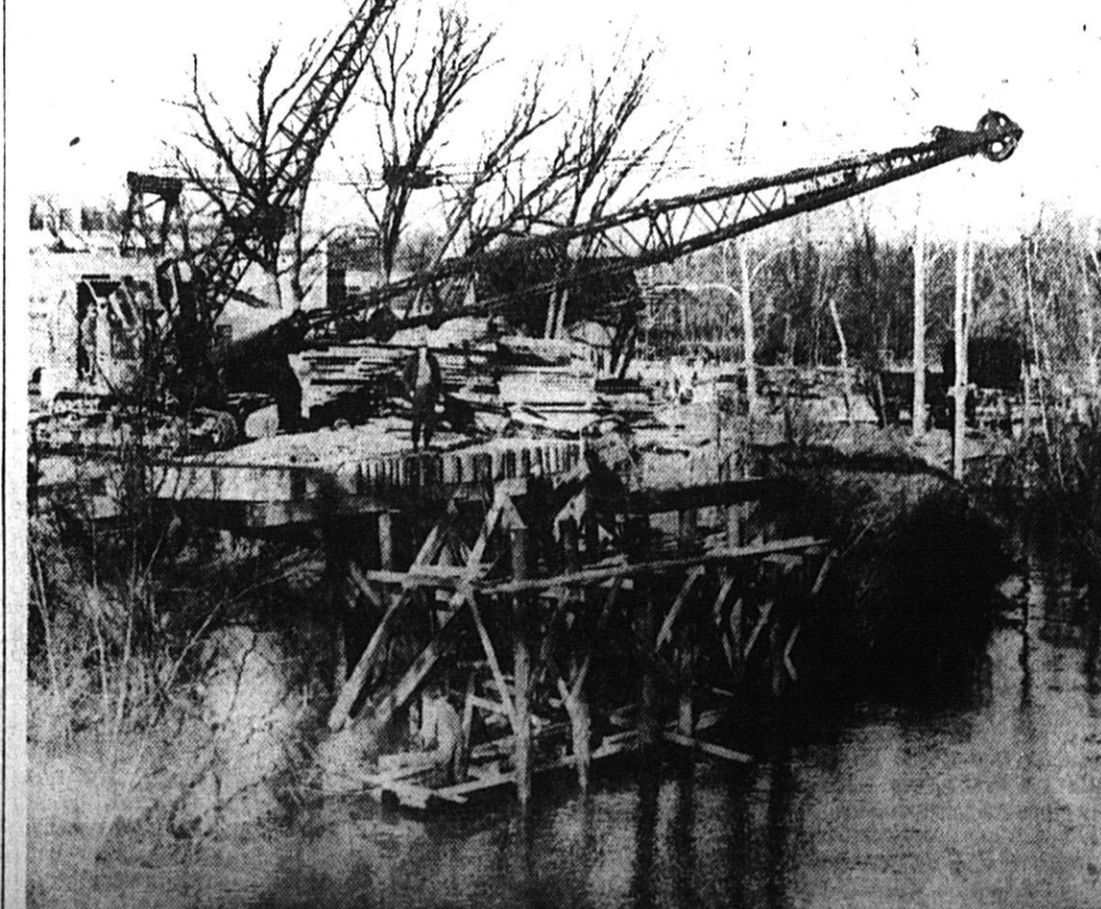
TEMPORARY BRIDGE TAKES SHAPE — Modern machinery and methods and rough hewn timbers and locally cut trees for piling provide a study in contrast as the temporary bridge to carry M-118 over the Kalamazoo River at Allegan takes shape. The bridge will be used to handle traffic while a new steel and concrete span is being built on the site of the present 65-year-old steel suspension bridge. Carl Goodwin and Sons, Allegan, are contractors.
