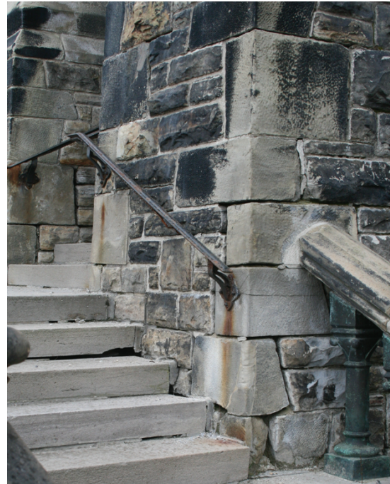
Figure 2. Loss of mortar in stone masonry due to freeze-thaw action.
