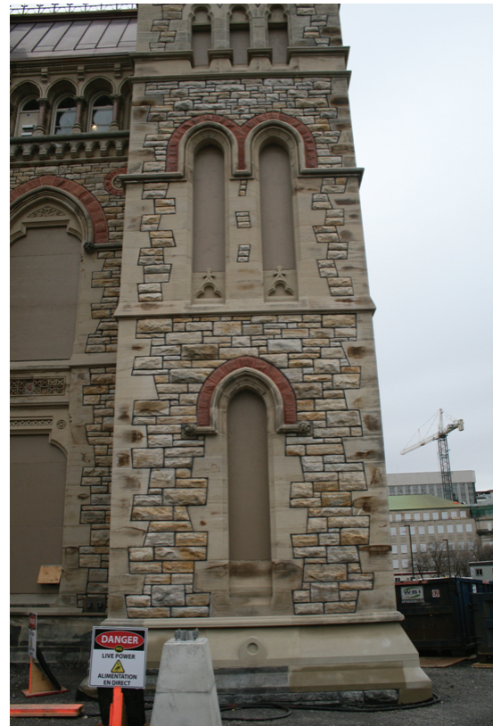
Figure 4. A section of the restored Westblock, on Parliament Hill, Ottawa. Note that the black mortar in the Nepean sandstone and the red mortar to match the red Potsdam sandstone above the windows follows photographic and written evidence that this was the form of the original construction.
