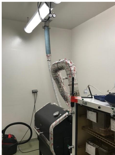
Figure 1. Electric smoker connected to central exhaust system
