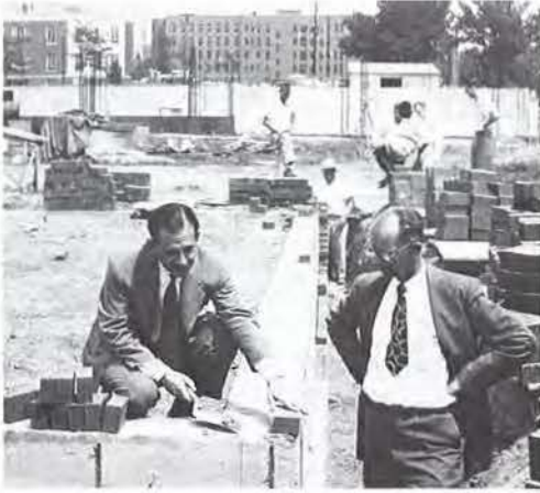
Drs. C. L. Wittson and J. P. Tollman at Nebraska Psychiatric Institute construction site, 1953.
