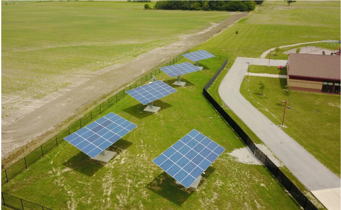
Figure 3.1: An installation of two-axis solar trackers at the Sheridan Community School
