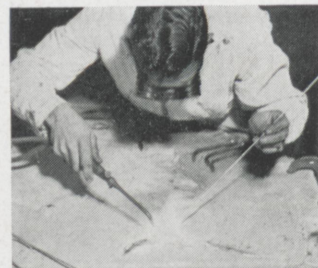
WELDING ALUMINUM—an architectural plaque, modern in design, is repaired by a modern method.
