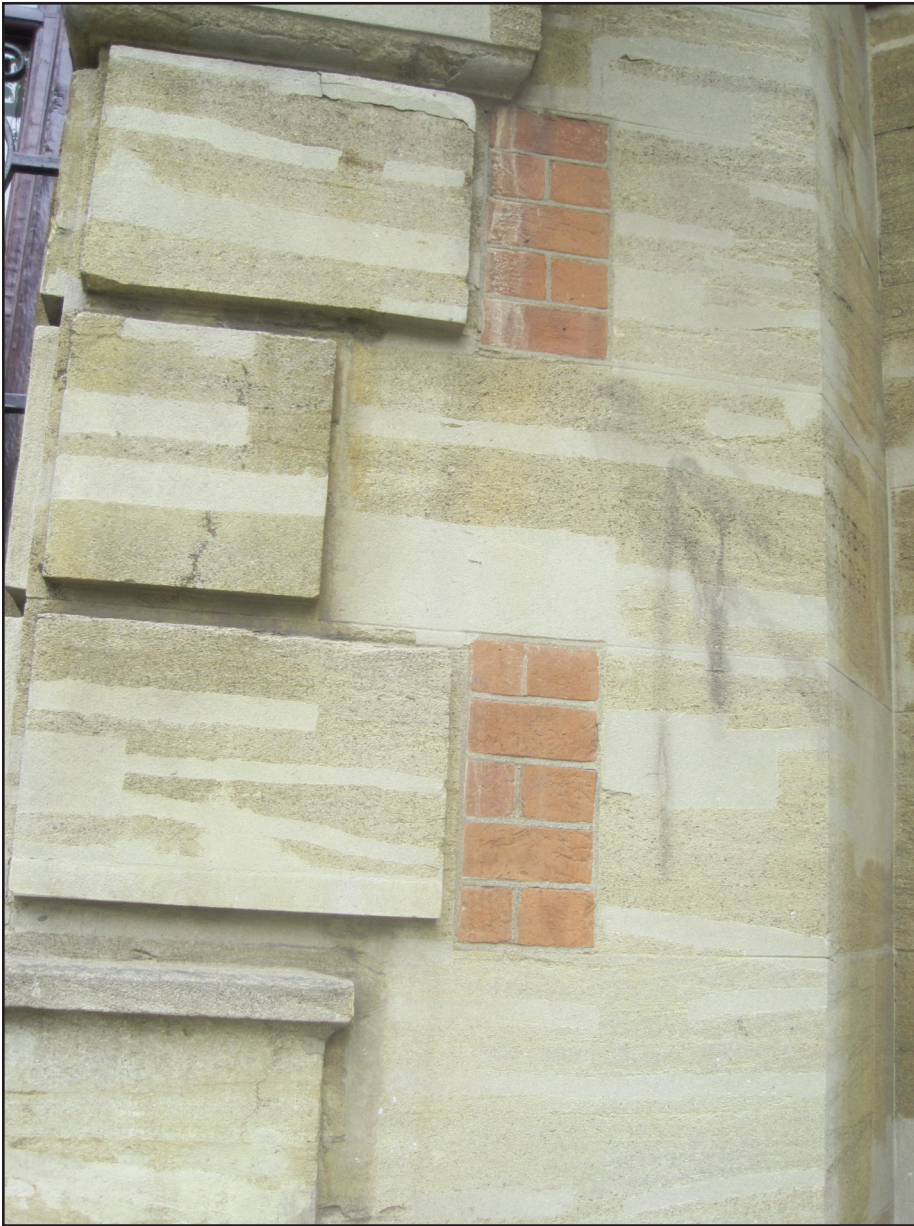
Figure 7. Part of the façade of a bank in Hampstead, London, showing inappropriate use of cement and brick in repairs to Douling Stone.
