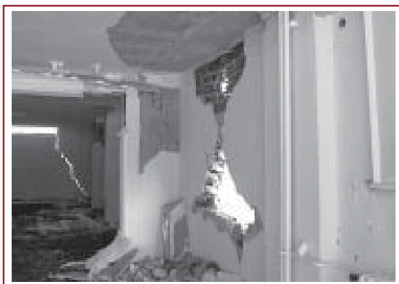
(b) Shear failure
