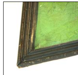
Figure 90: Frame surrounding the mural is in need of maintenance.
