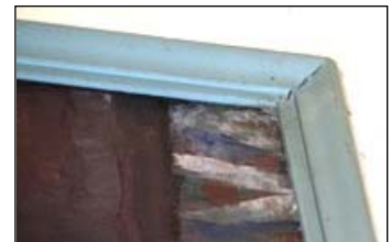
Figure 83: Frame maintenance is needed.
