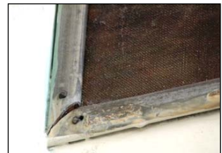
Figure 181: Deterioration of the frame surrounding the mural.
