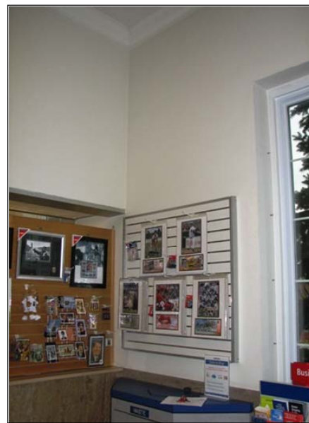
Figure 329: North wall of the post office and the adjacent corner; note that the moldings are original, suggesting that the original wall exists.
