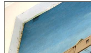
Figure 299 (right): The mural, which is recessed into the wall; the surrounding area shows signs of mold and dirt.
