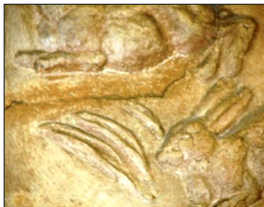
Figure 239: Detail of visible crack.
