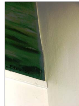
Figure 311 (right): Possible water and infestation issues.
