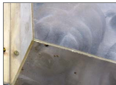
Figure 281: Detail showing grime and dirt possibly inside the encasement.
