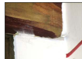
Figure 194: Separation of the canvas from the wall and wayward paint are visible.
