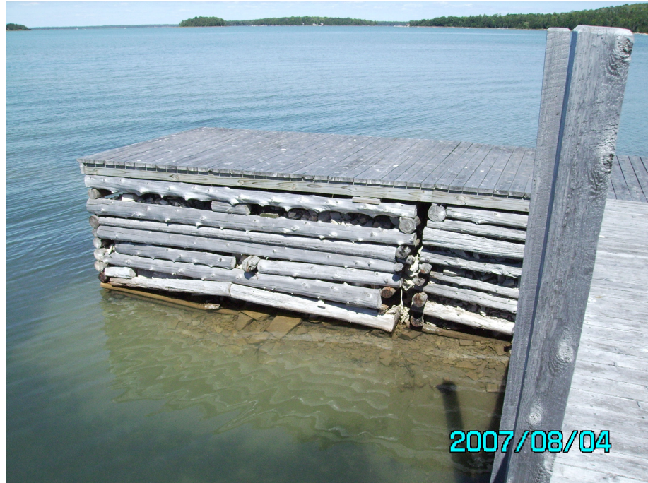
Figure 8. Dock Cribs Constructed with no Spacing Between Cross Timbers
