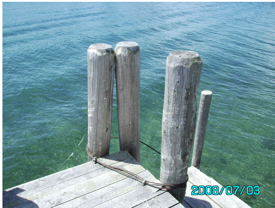
Figure 17. Dock End Piling Corner Cluster with Cable Reinforcement.
