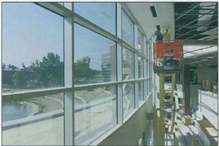
WINDOW VIEW: Work continues inside the new student center, which is expected to open Nov. 6. Here, a contractor works on the ceiling near the east side of the 181,000-square-foot building. Photo by Randy Mascharka
