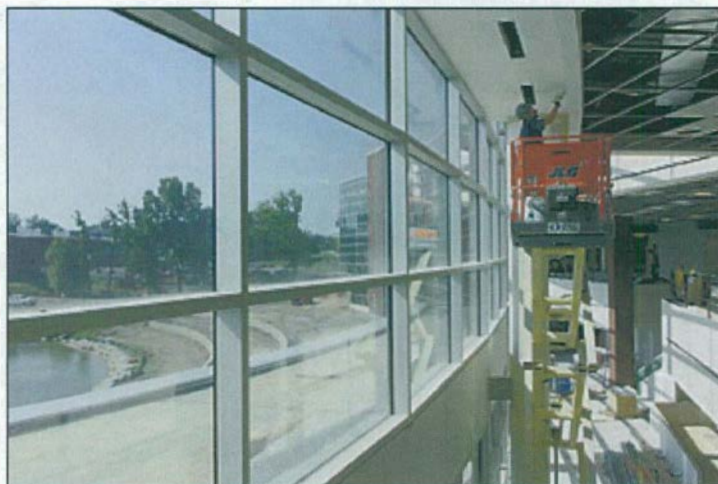
WINDOW VIEW: Work continues inside the new student center, which is expected to open Nov. 6. Here, a contractor works on the ceiling near the east side of the 181,000-square-foot building. Photo by Randy Mascharka
