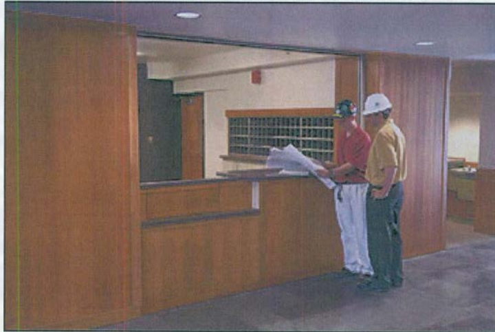
BUELL LOBBY: The Buell Hall lobby was renovated this summer, with work including a new front desk area. Here, Chris Longerbeam and Sean Berdan, coordinators of construction projects for the physical plant, inspect blueprints for the project. Photo by Randy Masharka
