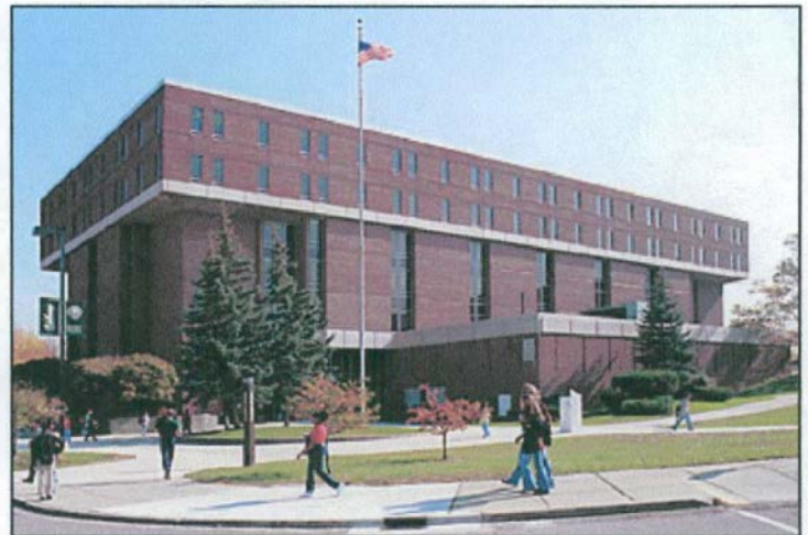
IN NEED OF CARE: Pray-Harrold, Eastern Michigan University's largest classroom building, is nearly 40 years old and in need of renovation. State legislators toured campus May 20 to learn more about the University's capital funding needs.
