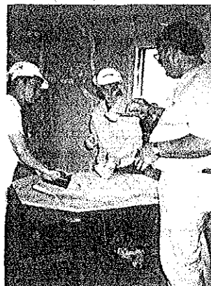
Andy Ladygo helping students prepare plaster for application on the interior of Building 3. Photo by Teresa Beagle.
