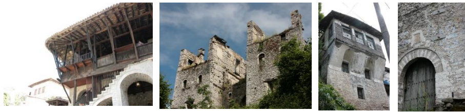
Fig. 5. Traditional Albanian crafts do not divide into masonry and carpentry: the sophisticated wooden roof structure of the Ethnographic museum house in Berat ( left ); horizontal wooden reinforcement of a double shell stone structure wall (Gjirokaster – center left ); lightweight upper floor in bondruk construction method (Gjirokaster – center right ); the arched doorway is probably constructed from foreign stone mason specialists, the metal work by local gypsies (Gjirokaster – right ); all photographs by Jaeger-Klein
