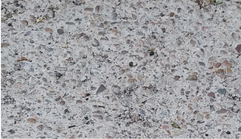
Fig 2: Deteriorated concrete surface at intersections
