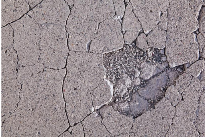
Fig 1: Deteriorated concrete surface due to aggregate expansion
