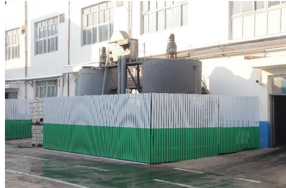
In this situation, the two chrome holding tanks are set in a sealed enclosure adjacent the tanning department.
