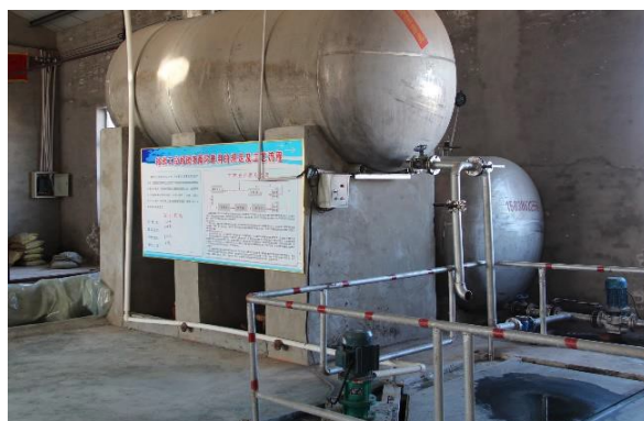
Tanks used for holding recovered chrome solutions with temperature adjustment via heat exchange. These are new to specification as shown, but are often adopted from other uses.
