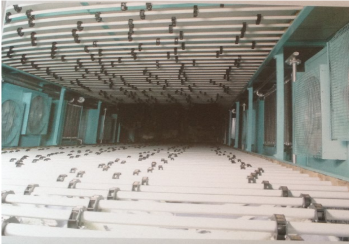
Fig. 4. A pole-drying tunnel (Source: Demaksan)
