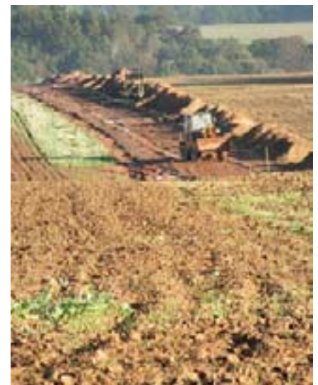
Construction of a rural lane in the Langenhessen cadastral district; photo: Langenhessen Community of Participants
