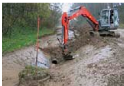
Exposure of piped sections of the brook; photo: Zschadraß (Hochwasser-) Muldedörfer Community of Participants
