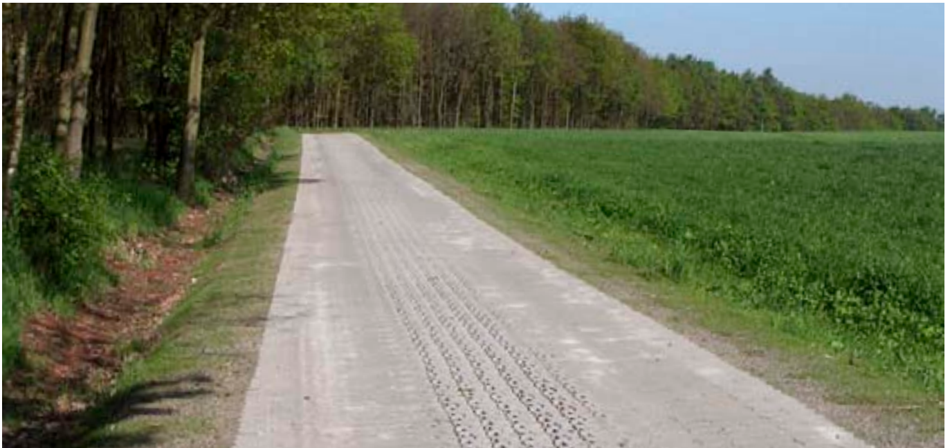
Expanded paved road in the Reichenbach-Falken land consolidation proceeding; photo: Reichenbach-Falken Community of Participants
