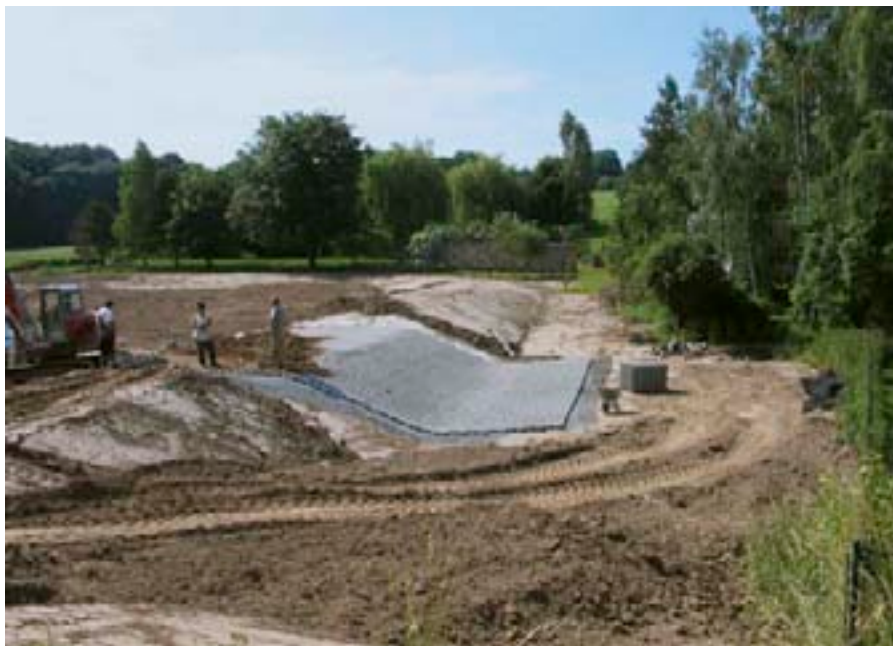
Construction of a fortified emergency overflow area for controlled drainage; photo: Zschadraß (Hochwasser-) Muldedörfer Community of Participants
