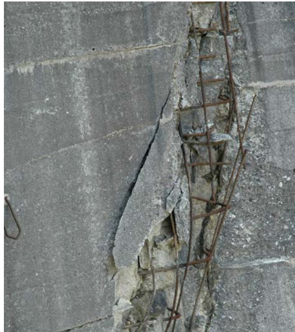
Figure 24: Rettenbachsperre: damage of steel reinforcement
