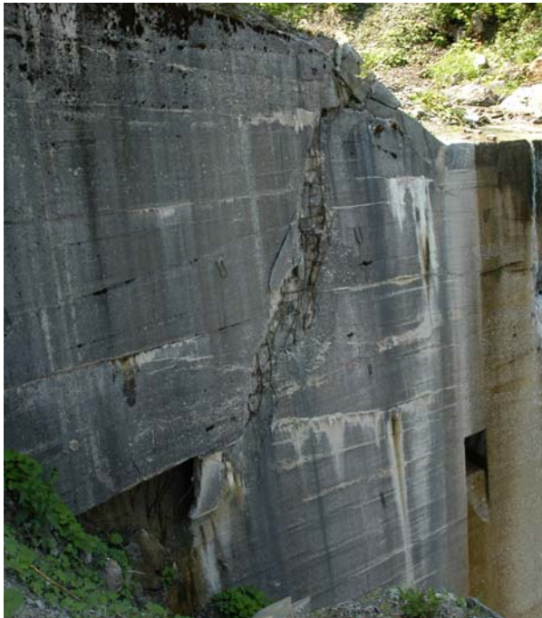
Figure 23: Rettenbachsperre: concrete damage due to rock thrust
