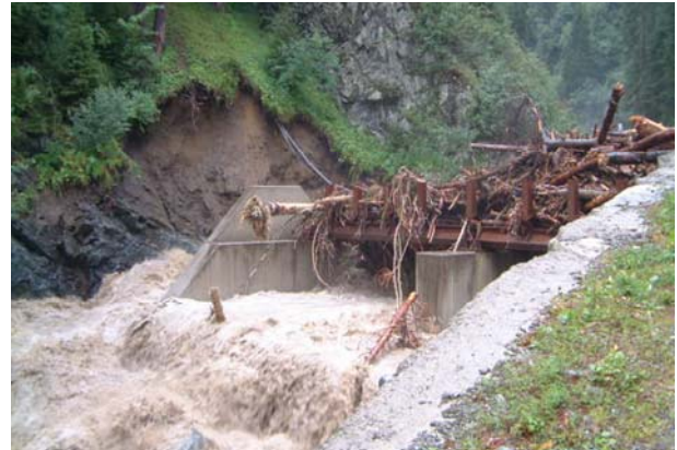
Lateral bypassing after clogging by woody debris
