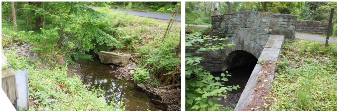
Gayley Run between Park Avenue and Ridley Creek Road (left); Gayley Run beneath bridge to Upper Bank (right) Photos: Walt Cressler, 2012
