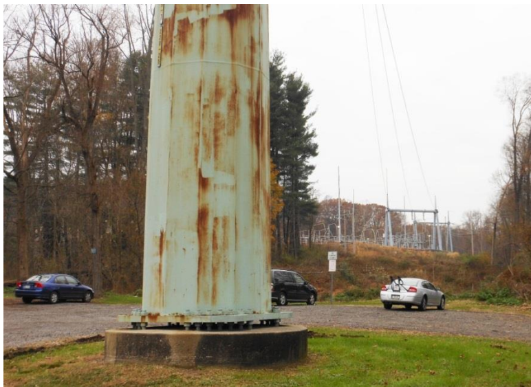
Power line pylon in the middle of Memorial Park parking lot Photo: Walt Cressler, 2012
