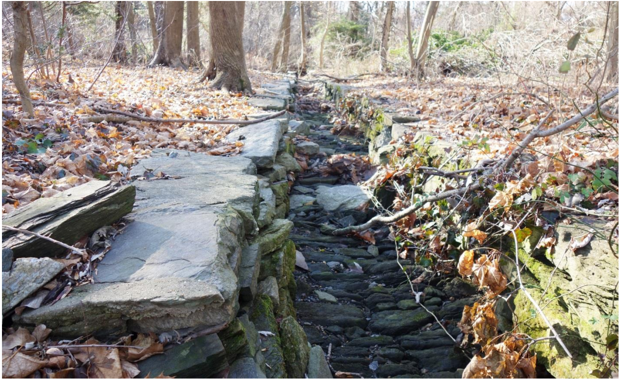
Reinforced stream next to Sproul springhouse/laundry, an unnamed tributary of Ridley Creek Photo: Walt Cressler, 2017
