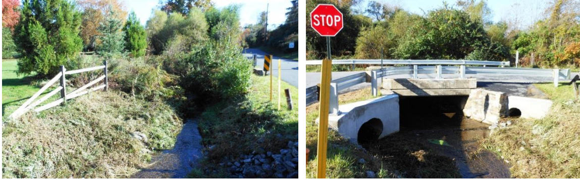
Two views of the stream at Stackhouse Mill and Valley Roads Photos: Walt Cressler, 2012
