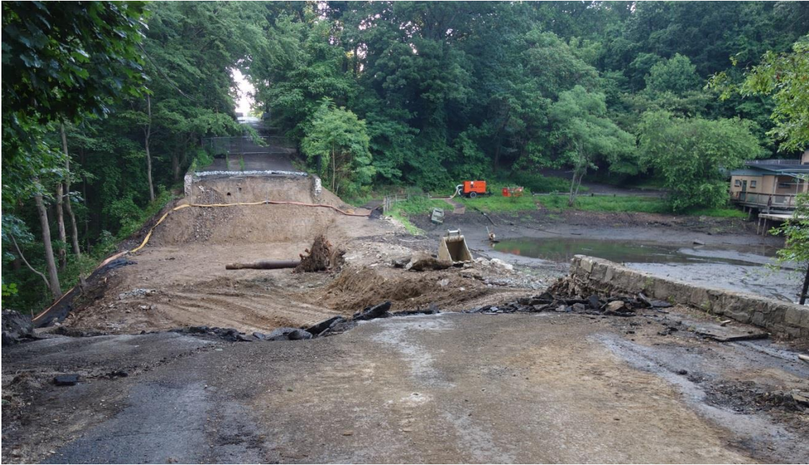
Broomalls Dam breach
