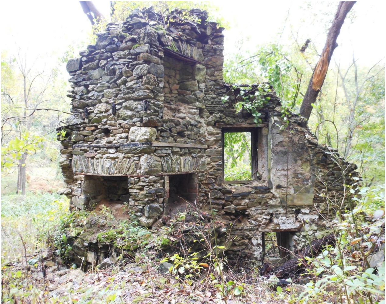
Ruins of millworker's tenant house along Multi-Use Trail Photo: Walt Cressler, 2012
