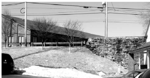
Figure 46. This stone wall is all that remains of the Chestnut Street bridge, which was replaced with the earthen fill seen to the left. Photo by the author.
