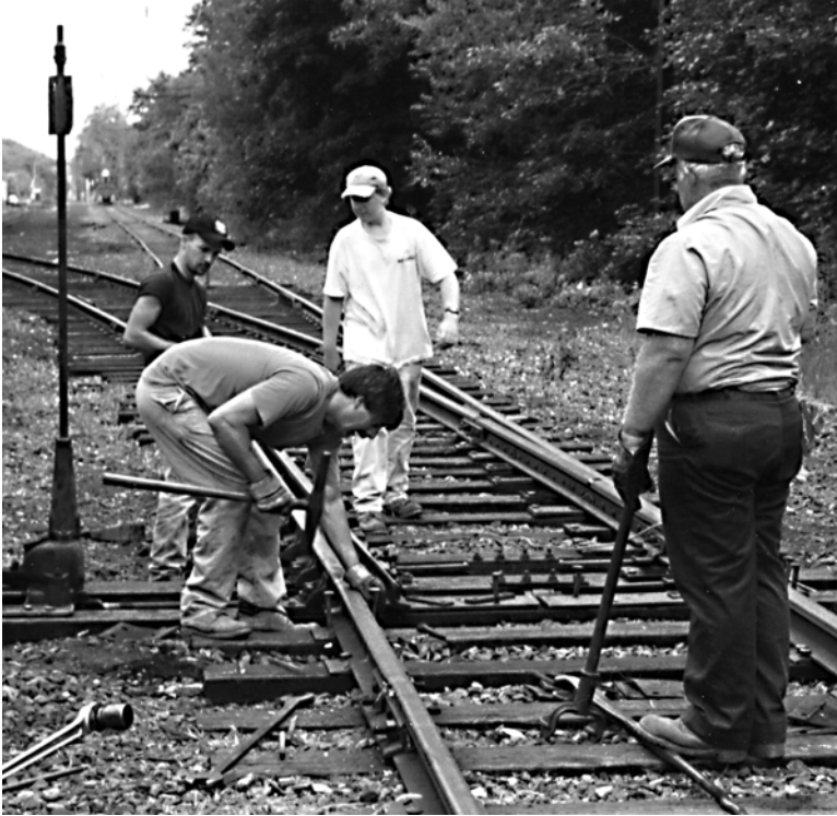
Figure 48. Skip Small supervises Joe Parsons, Bryan Small and another volunteer as they repair a switch near Union Street in 1998. Photo by the author.
