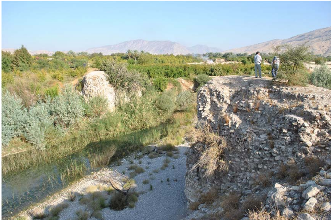
Fig. 37 - Bishapur, Fars province, a bridge (Pol-e Gabri) between Tang-e Čhowgan and the southern extremity of the city, photo MAI, by the author
