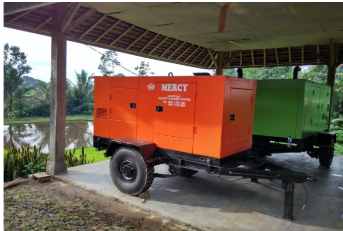
Gambar 9. Mesin Genset and Sound System
