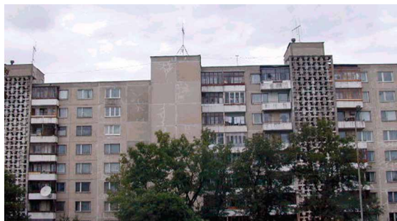
Figure 3.1. Damaged external walls of a panel house
