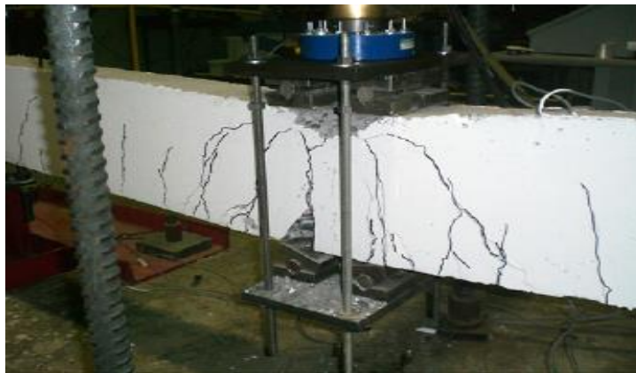
Figure 5-a. Failure condition of beam B2-SC
