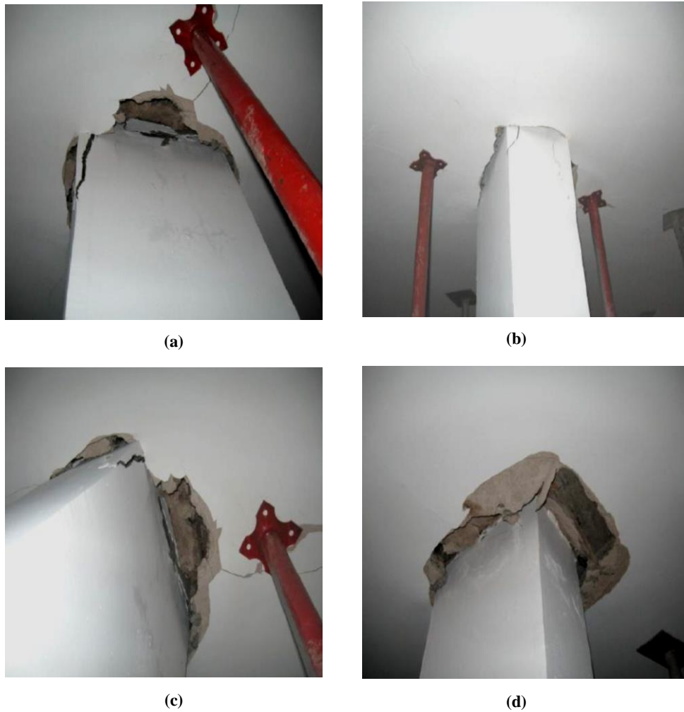
Figure 1. The punching shear failure in the case study (building in Baghdad)
