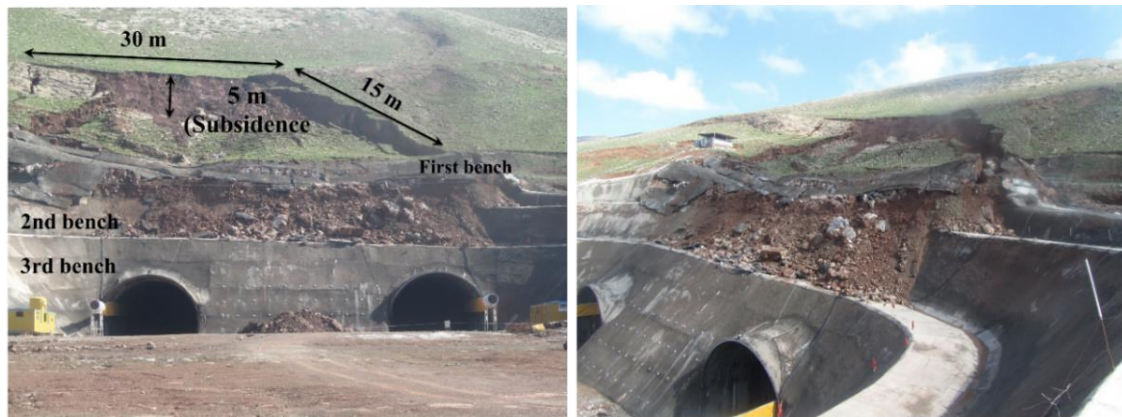
Figure 4. Subsidence of the Inlet Portal of Heybat Sultan Twin Tunnels
