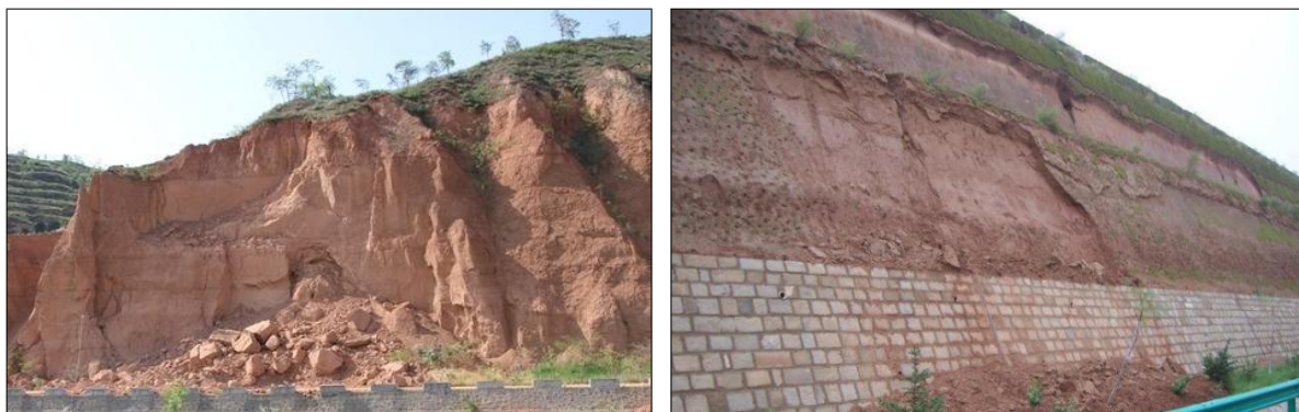
(a) Loess spalling hazards in Luo-chuan area
