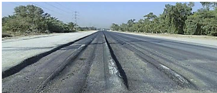
Figure 1. Shows rutting occurring in pavement (the road located in Iraq)
