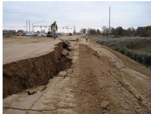
Figure 2. A 3.5-foot high scarp formed in the 15-foot fill over a 2-day period [1]
