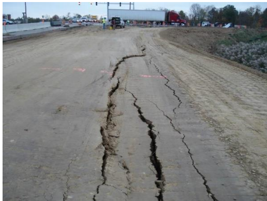
Figure 1. Shear Cracking begins in embankment fill at the end of fill placement activities [1]
