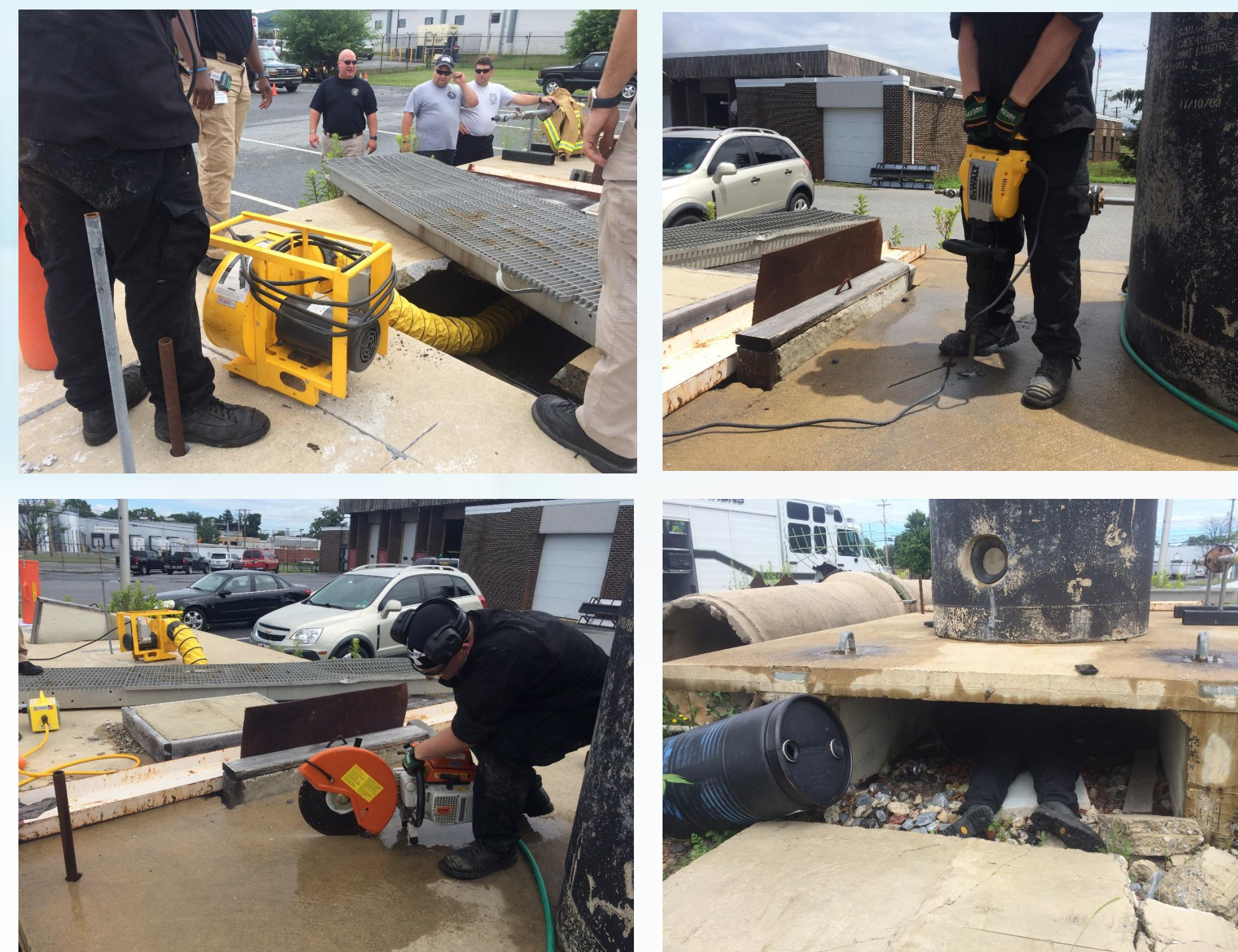
Fig. 1. Ventilation system (top left), demolition hammer (top right), K-12 (bottom left), confined space (bottom right)
