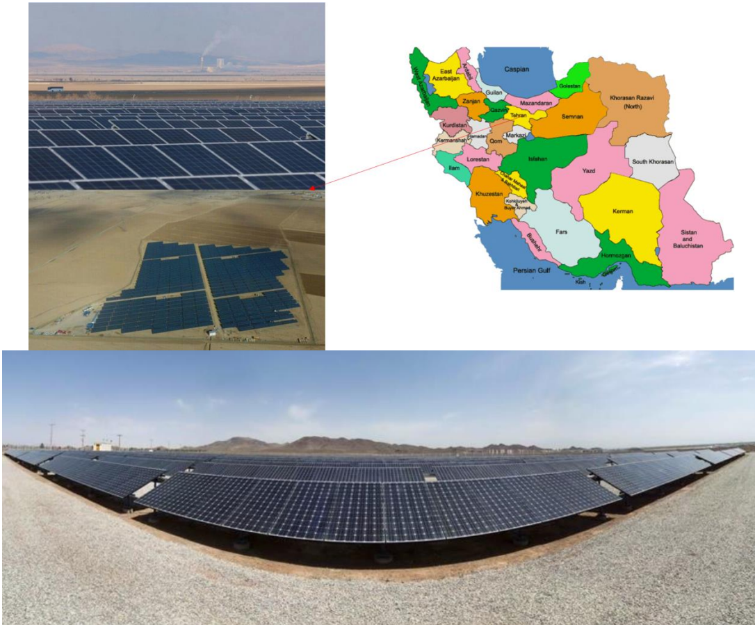
Fig -10: Atrin Parsian 2- Tehran solar power plant. [9]
