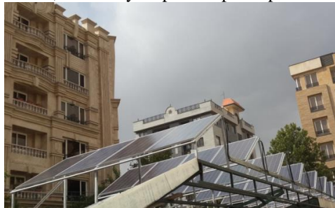
Fig -11: Solar panels of homes in downtown Tehran.
