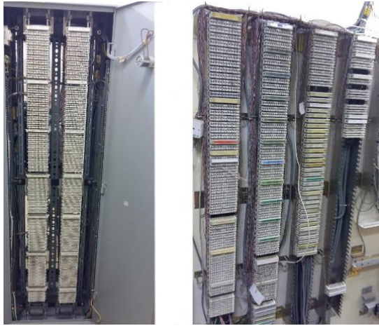
Fig. 1c. Digital Distribution Frame (DDF) and Main Distribution Frame (MDF). Left – installed in the cabinet, right – wall-mounted open panel.
