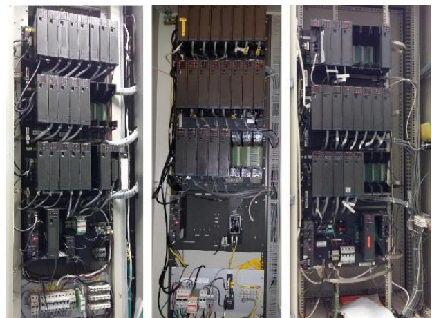
Fig. 1b. MOSCAD-RTU cabinets
