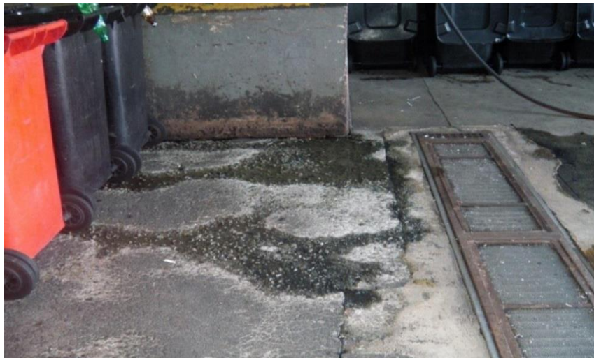
Figure 4.12 Damaged concrete flooring
