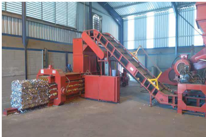
Figure 5. Refuse-derived fuel plant at Interwaste recycling hub
